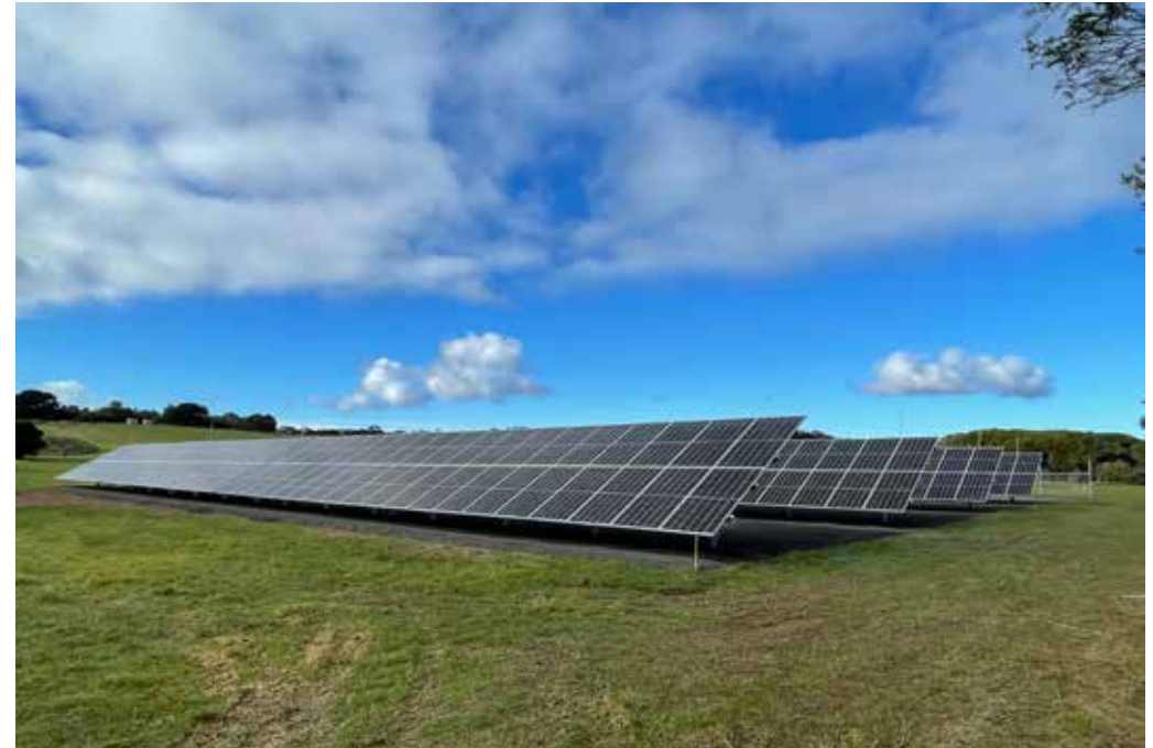
Solar panels at our treatment plant
