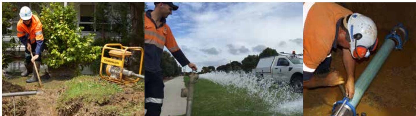
Left: Work crew responding to burst main. Middle: Maintenance crews flushing water supply. Right: Emergency repairs.
