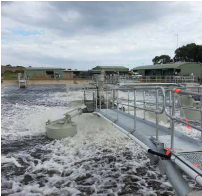
Caption: Cowes Waste Water Treatment Plant.
