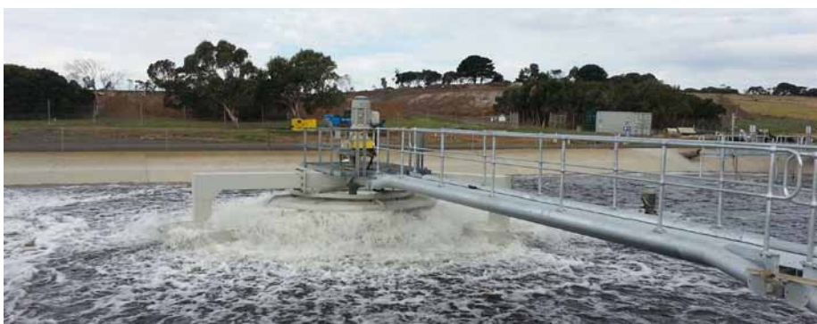
Cowes Wastewater Treatment Plant
